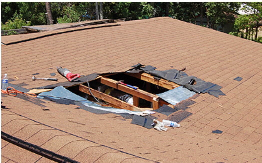
The problem roof
