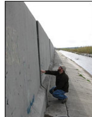
Louisiana State University researcher Ezra Boyd examines a crack in a flood wall in Jefferson Parish, west of New Orleans. Scientists say many levees that survived Hurricane Katrina are compromised and may fail in another storm. (By Joby Warrick -- The Washington Post)
