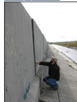
Louisiana State University researcher Ezra Boyd examines a crack in a flood wall in Jefferson Parish, west of New Orleans. Scientists say many levees that survived Hurricane Katrina are compromised and may fail in another storm. (By Joby Warrick -- The Washington Post)
