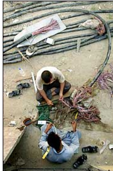
Justin Lane for The New York Times Work is under way to rebuild Baghdad's telephone system, a crucial part of getting Iraq back on its feet. Each line must be spliced and tested.
